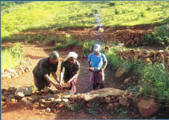
Terracing of FRA Lands under NREGA Work: Kebedi, Rayagada – an outstanding example of convergence
